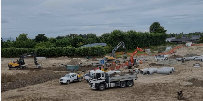
Drainage and pumps
